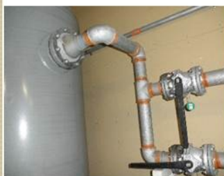
Large-bore pipe and receiver tank with adequate capacity
