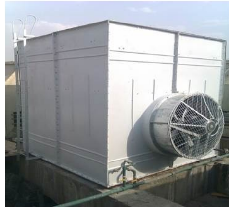
Forced Draft Cooling Tower
